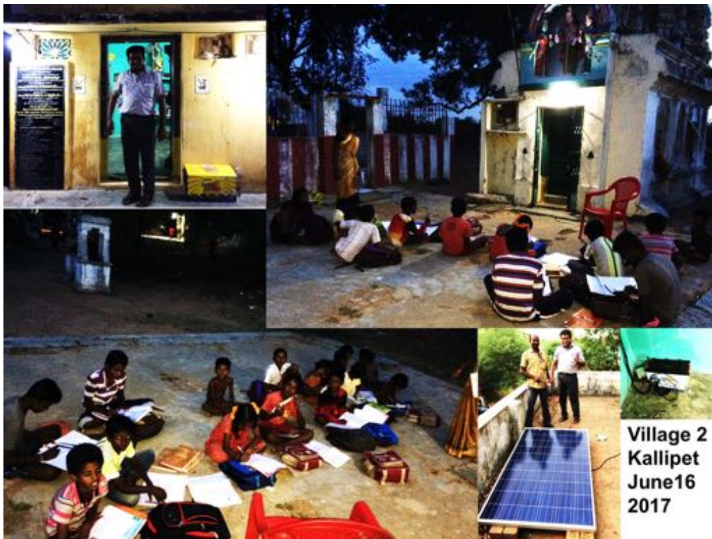
Figure. 16.3: Second PV system installation: Kallipet, June 16, 2017. Courtesy Augur Computers and Swami Vivekananda Rural Development Society.
